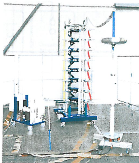
Impulse test system SGSA 900 kV, 45 kJ
